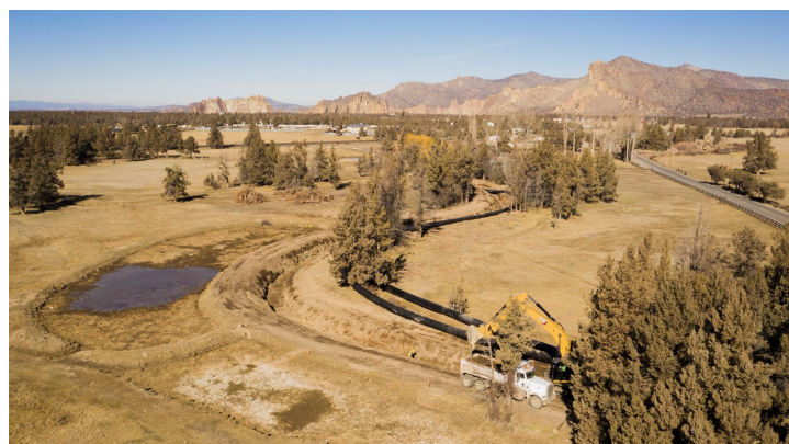
Central Oregon Irrigation District: Construction of Smith Rock Pipeline. Photo credit FCA.
